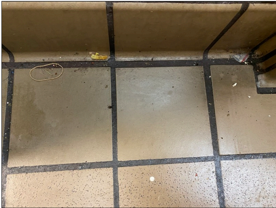
6 - HA-06: Non-ACM black tile grout in BOH
