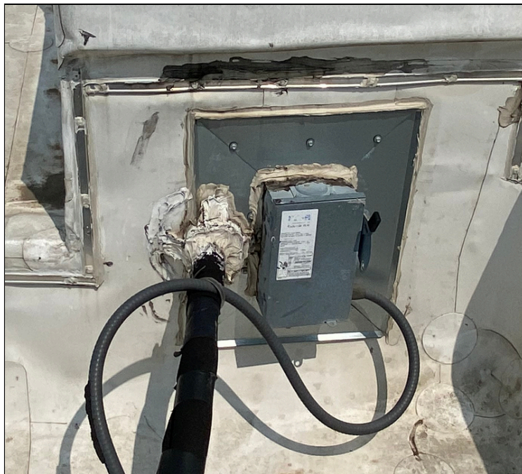
12 - HA-12: Non-ACM white caulk on roof penetrations
