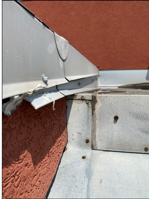
11 - HA-11: Non-ACM light gray caulk on cooler roof
