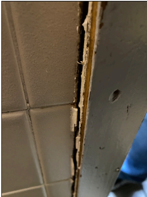
8 - HA-08: Non-ACM white caulk around BOH interior door frames and at FRP panel seams
